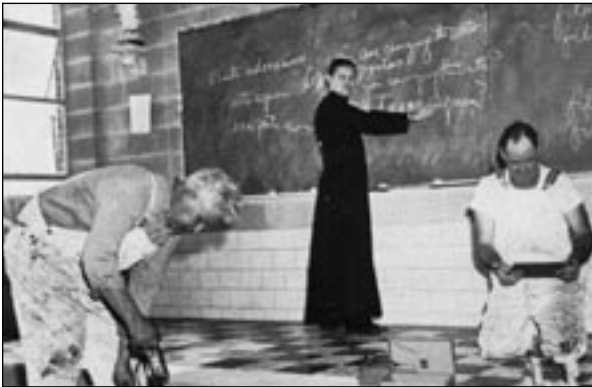
Brother Peter L. Lawrence teaches while the construction goes on around him.
